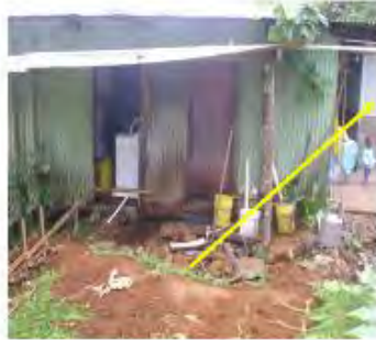
Bathroom relocated from back to side of Building. Old bathroom was not accessible for Roy with rocks used as flooring, not properly concreted
